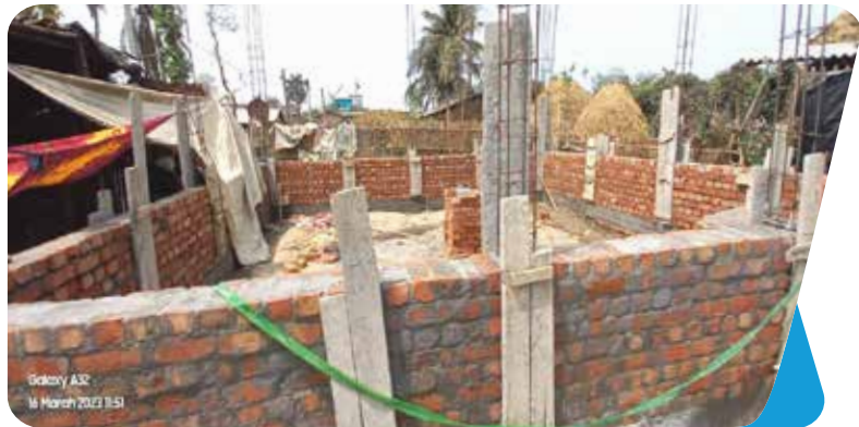
Construction work of pucca house with the provision of two rooms, kitchen, toilet and bathroom
